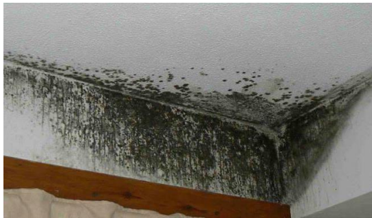
Damps on wall and ceiling surfaces
