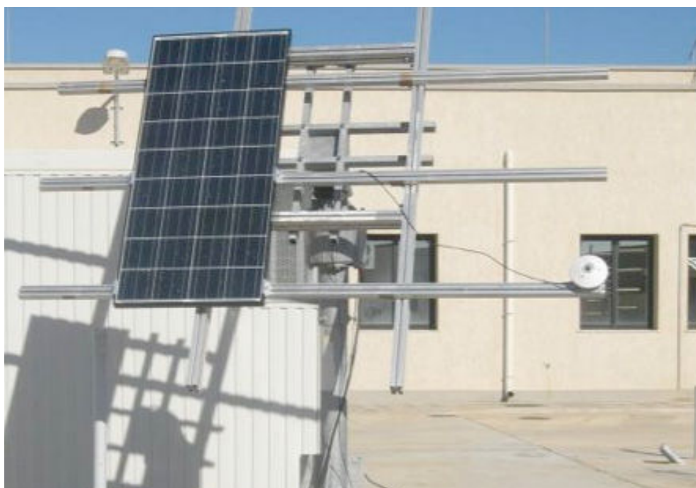
Figure 30: CSERS Solar PV Conversion Lab
