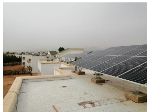
Hayah Regency 152 kWp
