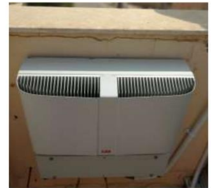
Limitation of space, inverters with direct sunlight
