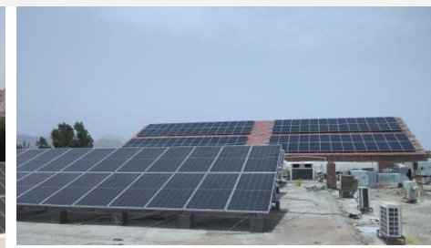
Regency Palaza 126 kWp
